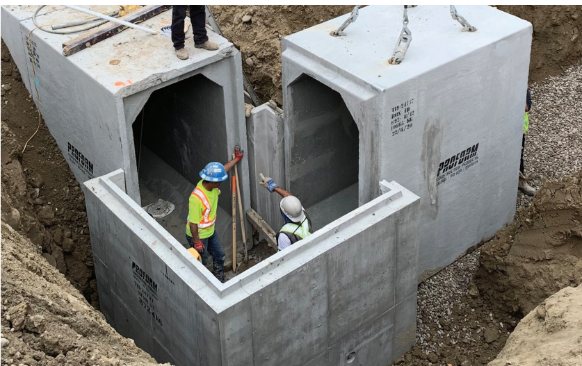
Maintenance hole and culvert connection
